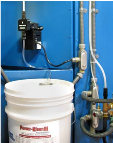
Typical Rinse Chemical Injector Pump mounted on MART
